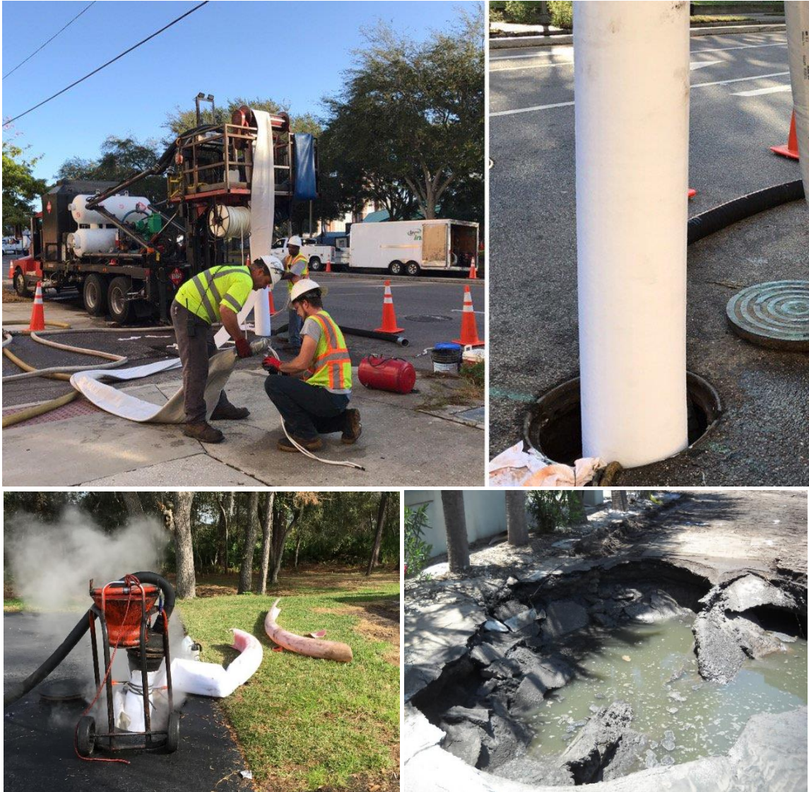
Figure 4-2. Top left, top right, and bottom left show pipe rehabilitation efforts to combat the aging infrastructure within Pinellas County. Bottom left image shows the result of a broken main.
