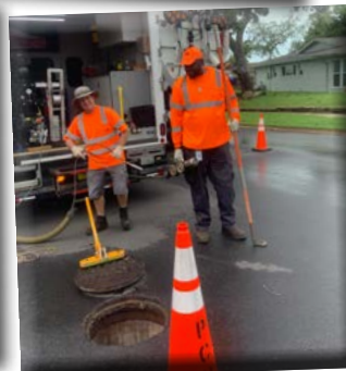
Utilities employees Raymond Wells (left) and Kedrick Poole (right) inspect a sewer line in Largo ahead of the storm
