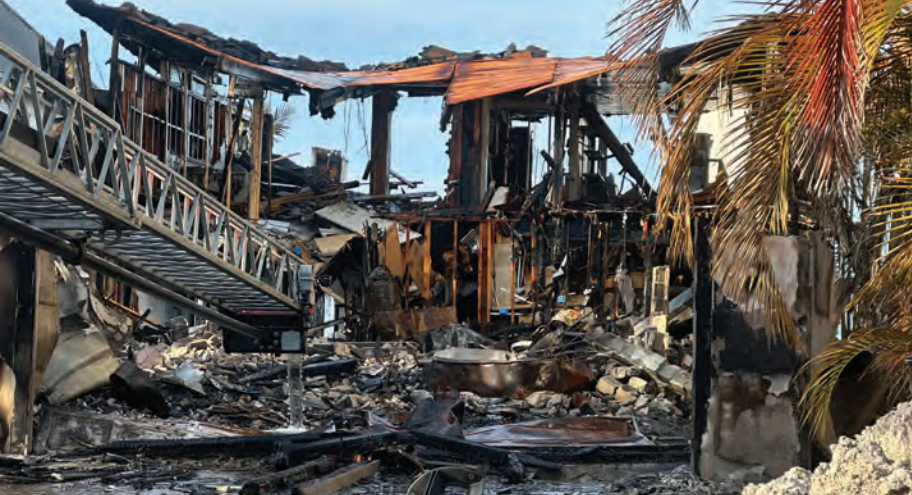
A beachfront home is left destroyed by a fire during a storm.
